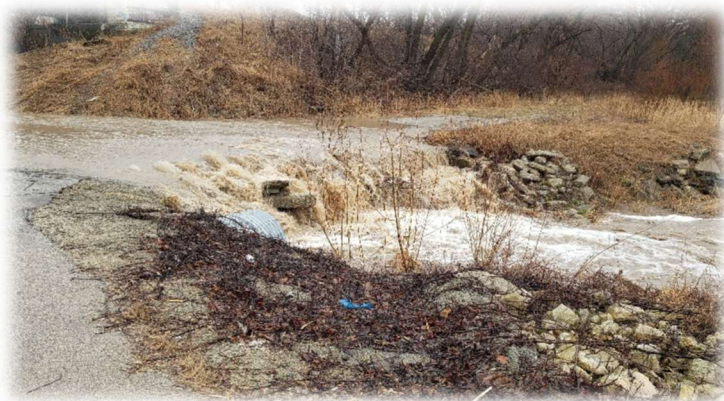
Flooding at 67 th Drive
